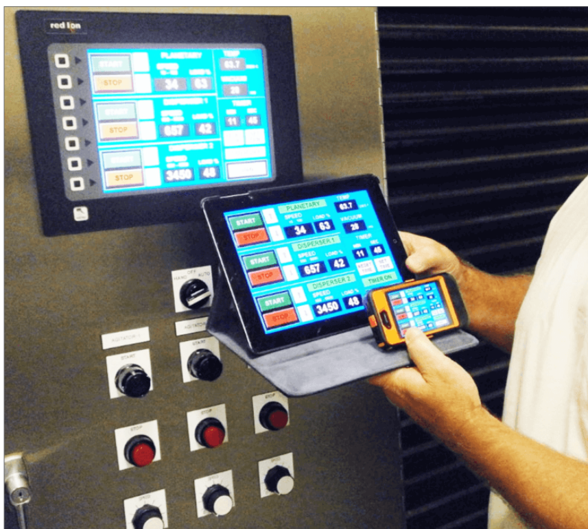
ROSS control system
