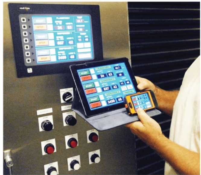
● Figure 3. Programmable logic controller
