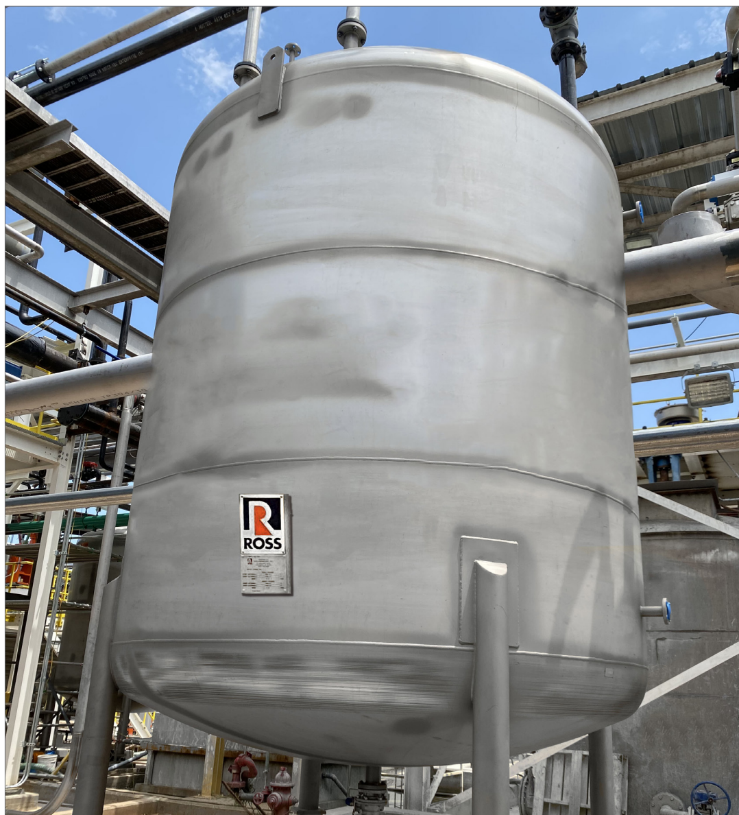
ROSS 9,400-gal condensate receiver tank is designed and built according to ASME standards for up to 5 psi at 200°F.
