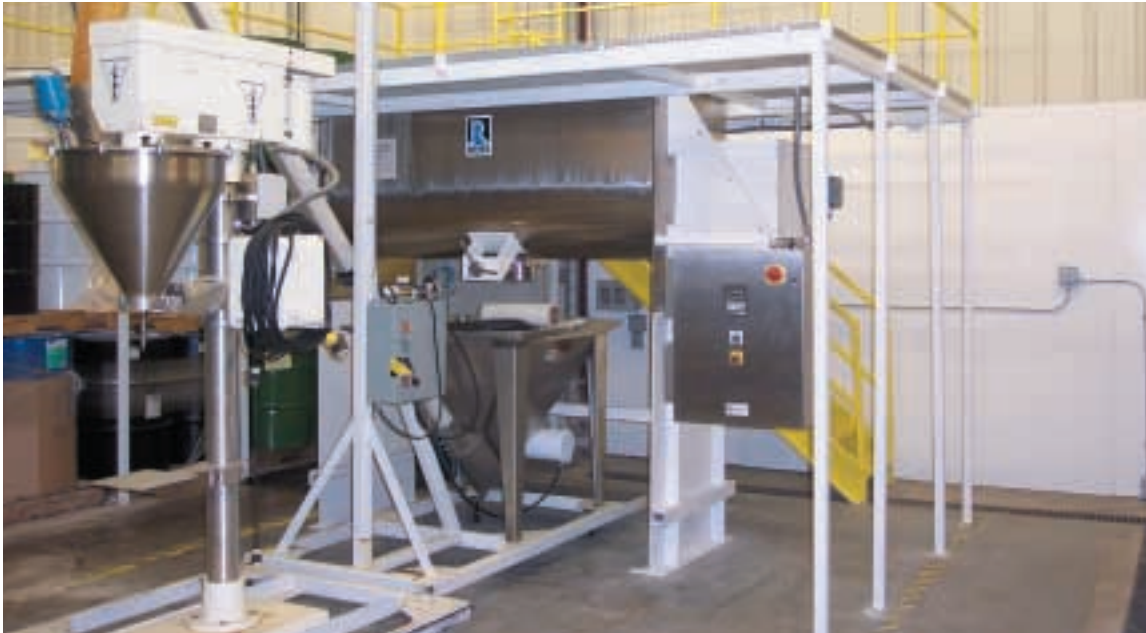
The elevated sanitary Ribbon Blender installed in the GloryBee facility is positioned to discharge directly into an auger filling/dispensing system below. The panel at right provides both start/stop functionality as well as variable speed control.
